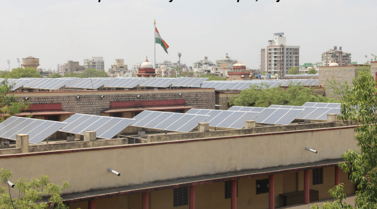
Roof-top Solar PV System in Jaipur, Rajasthan
